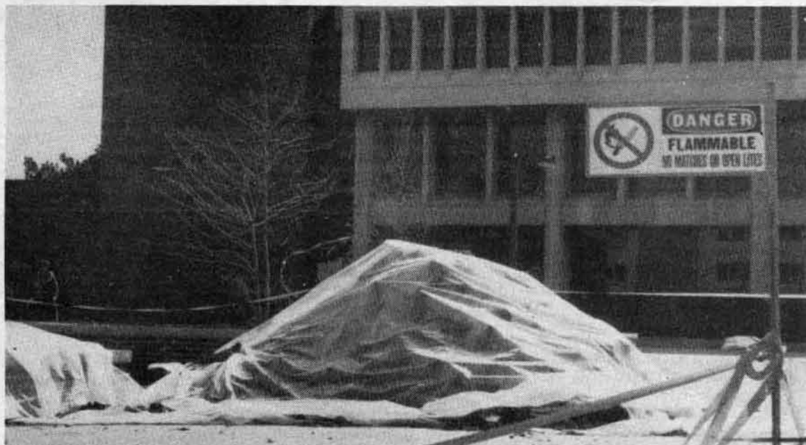
DIGGING FOR TREASURE?: That dirtpile in the quadrangle has unearthed nothing more mysterious than a faulty gasline in need of repair. [Photo by D.K. DeIermann.]
